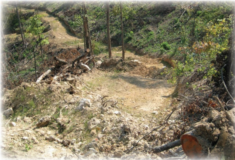
Figure 1 (above): When skid trails are no longer in use any ruts should be removed and permanent water control structures such as water bars installed. Skid trails that are erodible should be seeded to initiate grass cover.
